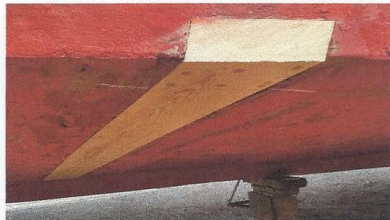
First and only bottom plank replaced in 26 years. 6 inch stainless steel ring nail fasteners are hidden behind the wooden plugs
